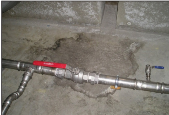
Leaking fittings are due to low-density PTFE Tape.
